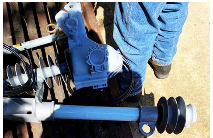
Fig. 4 New PG&E Insulators
