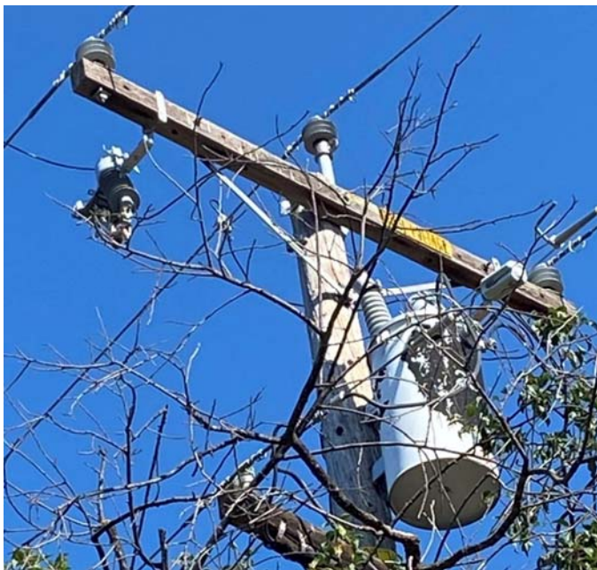
Figure 6 New insulators on top of the power line pole.
