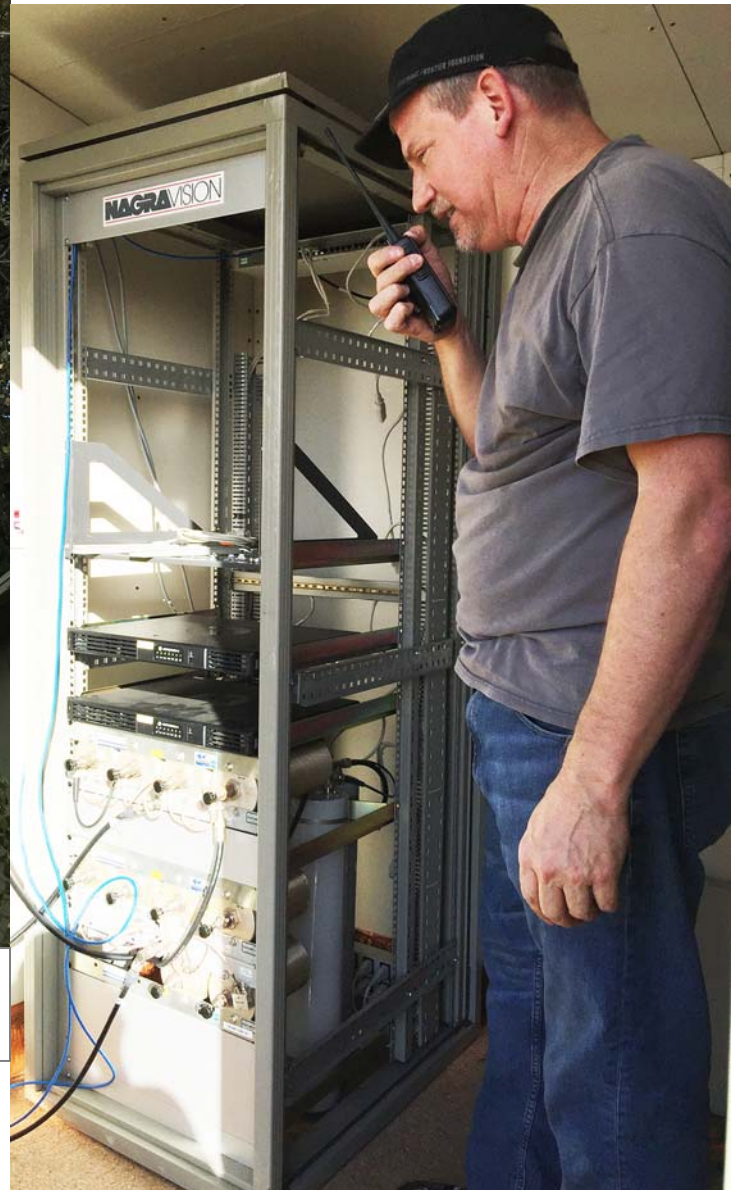
Joel is testing the repeater after the repeater equipment was re-racked into a larger equipment rack to make room for more exciting things to come.
